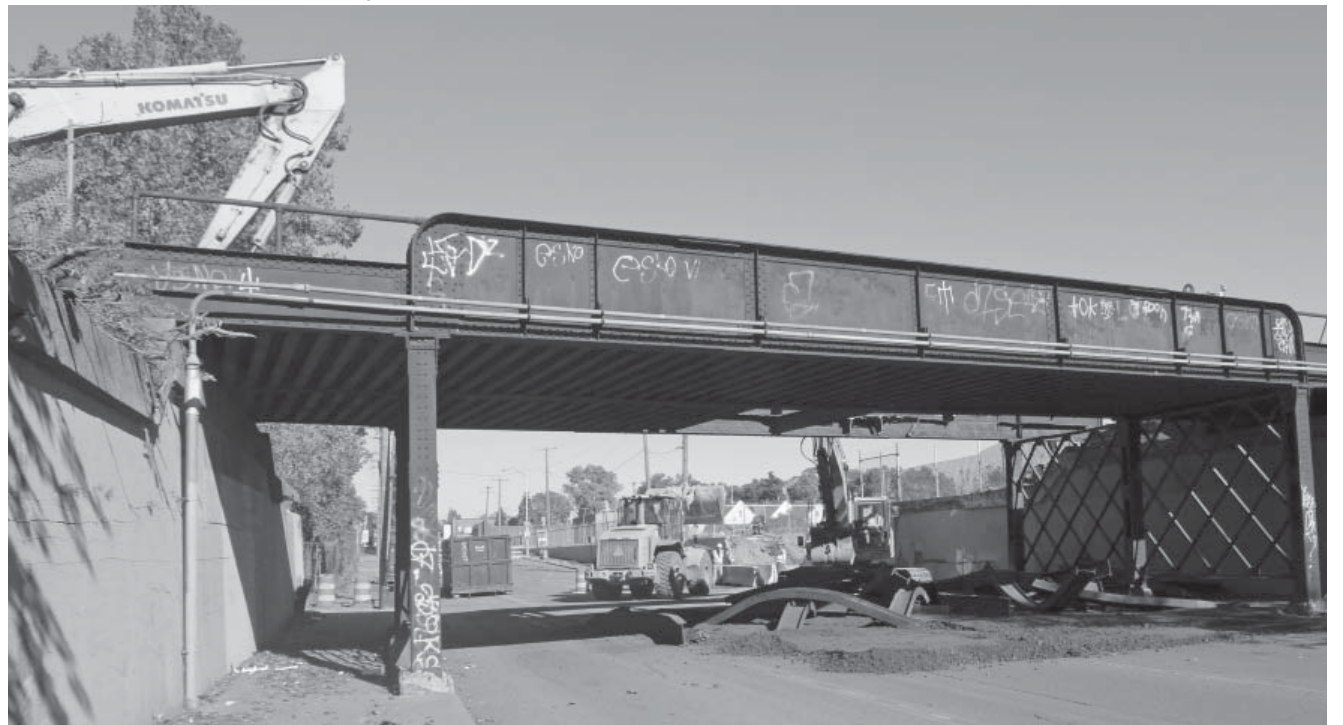
It took one day to demolish the old bridge over Junction Ave. in Detroit. (Photo by Steve Sobel)
