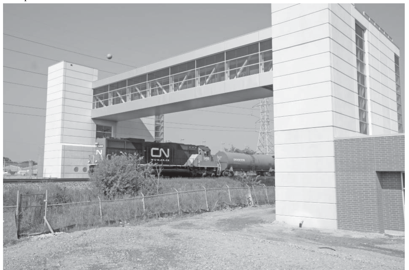
ALMOST DONE. A CN freight train passes underneath the walkway to passenger boarding platform at the new Troy Transit Center. Construction at the center continued last summer despite continued legal fights over ownership of the property. In May, the Michigan Court of Appeals ruled that the developer of an adjacent shopping center has title to the transportation center land. The city of Troy and Grand Sawka Properties have been fighting over the transit center property since 1999. The city has appealed the latest ruling to the Michigan Supreme Court, and has begun preparations for condemnation proceedings. (Photo by Steve Sobel.)
