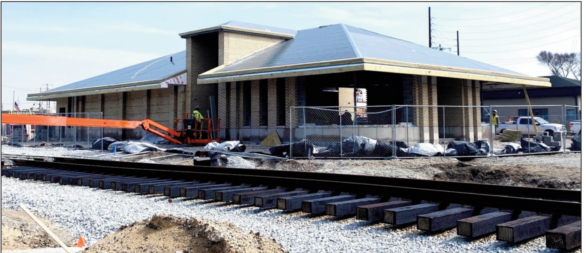
The New Miller Road Station in Gary is under construction as part of the double tracking improvements to the South Shore Railroad. (NICTD Photo)
