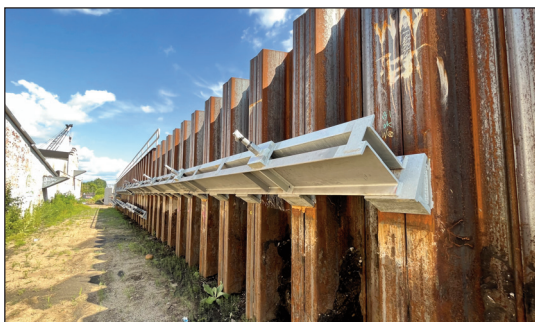
Looking east at the new sheet pile retaining wall along the north side of the railroad west of Jackson Street.
