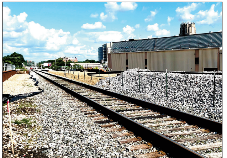
Looking east at the west end of the Jackson Street Bridge. The south track (on the right in the photo) has been raised 3 to 4 feet to allow the bridge to be raised by this amount to increase the clearance over Jackson Street to about 14 feet.
