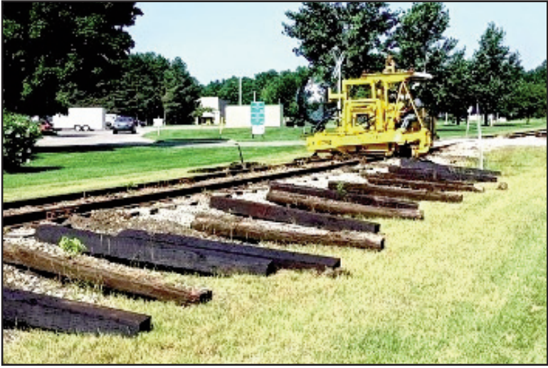
Tie replacement project on the railroad which is owned by MDOT and leased to Great Lakes Central Railroad.
