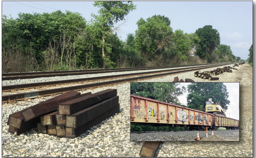
Staged ties and tie train; part of the ongoing track work on the Michigan Corridor at Jackson, which will include raising the tracks a few feet as part of the replacements of two bridges. (JHG photos)
