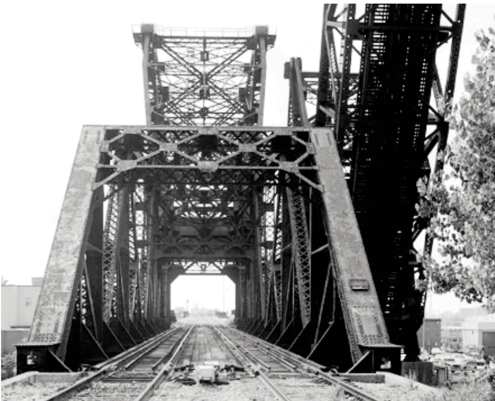
Looking west from the east side of the Chicago River at the deck of the SCAL Bridge. The SCAL remains in daily use for freight and Amtrak passenger trains. According to Wikipedia, the adjacent raised bridge, was built by the Baltimore and Ohio Railroad in 1930. It is no longer used and was part of another elevated double track line that crossed the north-south railroads and the river to former freight yards and passenger yards at Central Station to the northeast (behind the camera). (Library of Congress photo)
