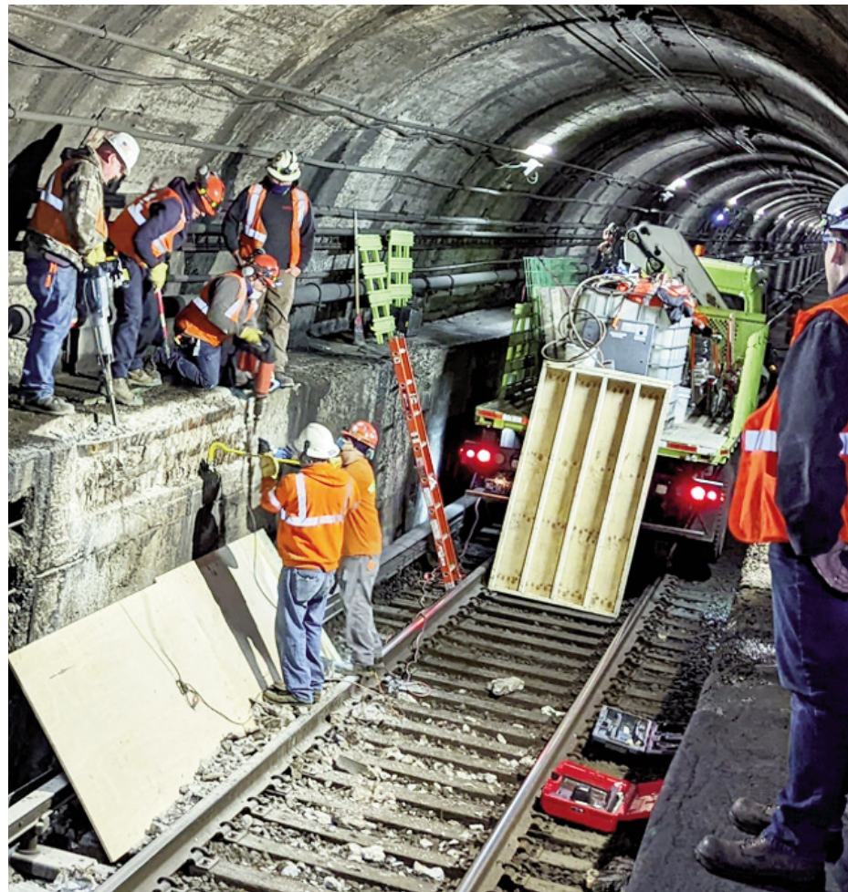
Amtrak has been taking a series of 55-hour outages on weekends to make repairs to the North River Tunnel under the Hudson River leading to Penn Station in New York. The work involves repairs to the masonry surfaces, electrical lines, and the signal system in an effort to reduce leakage and ensure the continued safety and reliability of the tunnel. (Amtrak photo)
