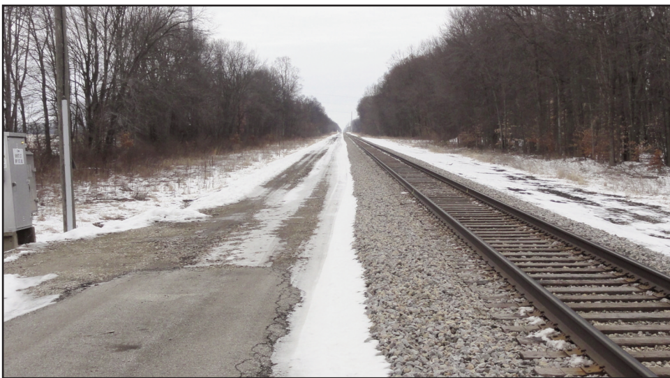
Looking east from White Street (east of Niles) showing the existing right-of-way with space on the north (left) side for a second track. This was previously a double-track railroad. (Jack Kessler Photo)
