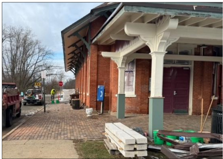
Masonry repairs are being performed by Bonnor Restoration Company to the exterior walls of the Amtrak Station in Albion. Work started in late 2024 and includes replacement and re-pointing of brick along the base of the exterior walls. The building, built in 1882, by the Michigan Central Railroad, was abandoned until saved in the 1980's by Albion's Cran Family. The structure serves a small number of daily Amtrak and Greyhound passengers. (Matthew Murawski photo.)
